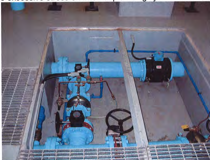
Figure 5 – Zone 4 Pump/Pressure Reducing Station on 30 th Street NE
