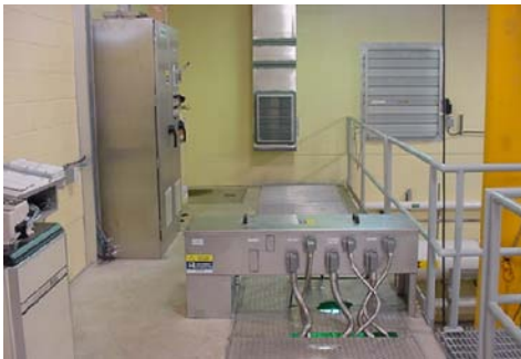
UV Treatment System
