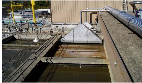
Primary Sedimentation Tanks
