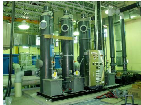
Train B Odour Scrubber
