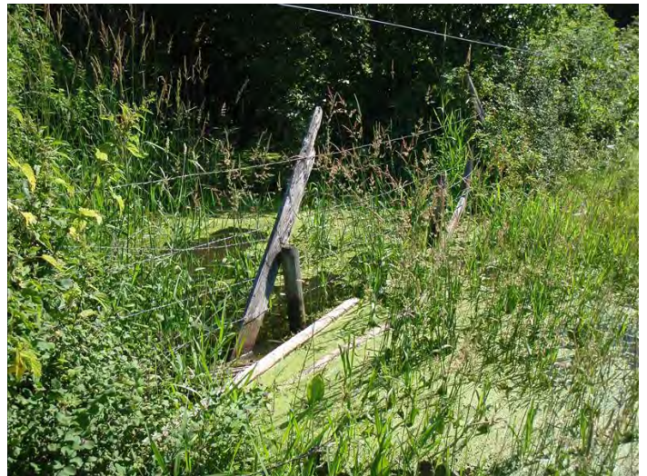
South Rumball, Segment 4, Obstruction Point 3
