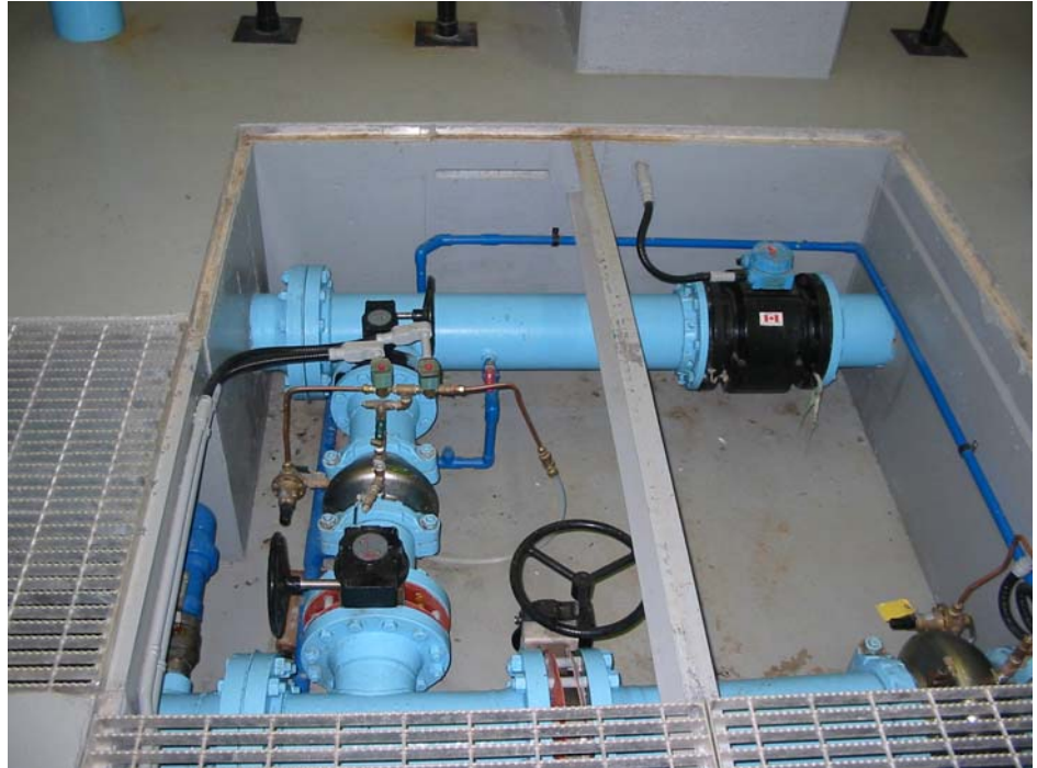
Figure 4 – Zone 4 Pump/Pressure Reducing Station on 30 th Street NE
