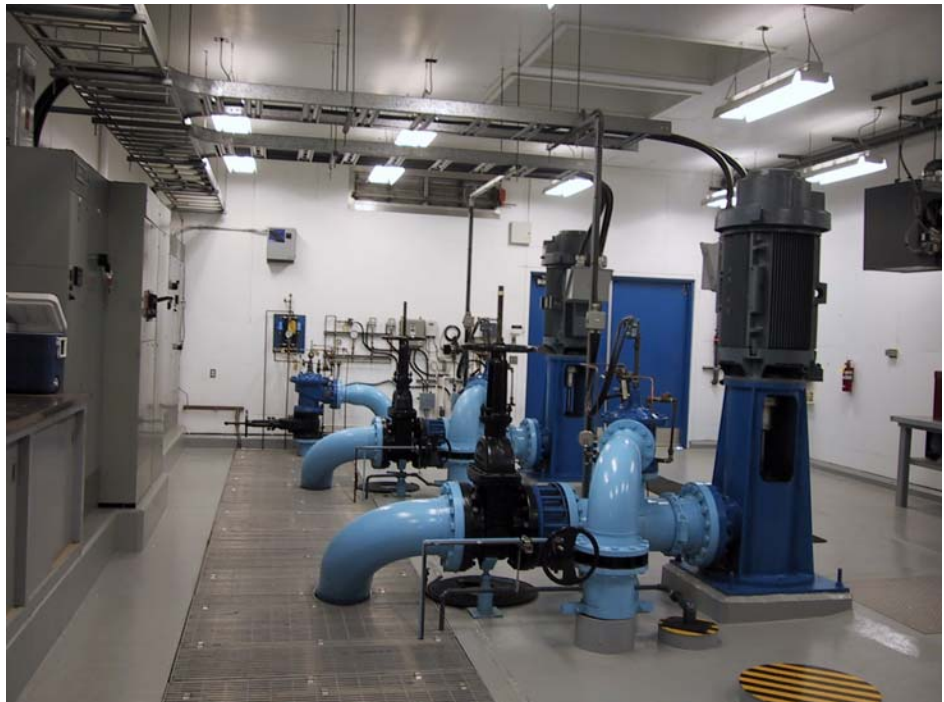
Figure 3 - Zone 1 Pumping Station at Canoe Beach
