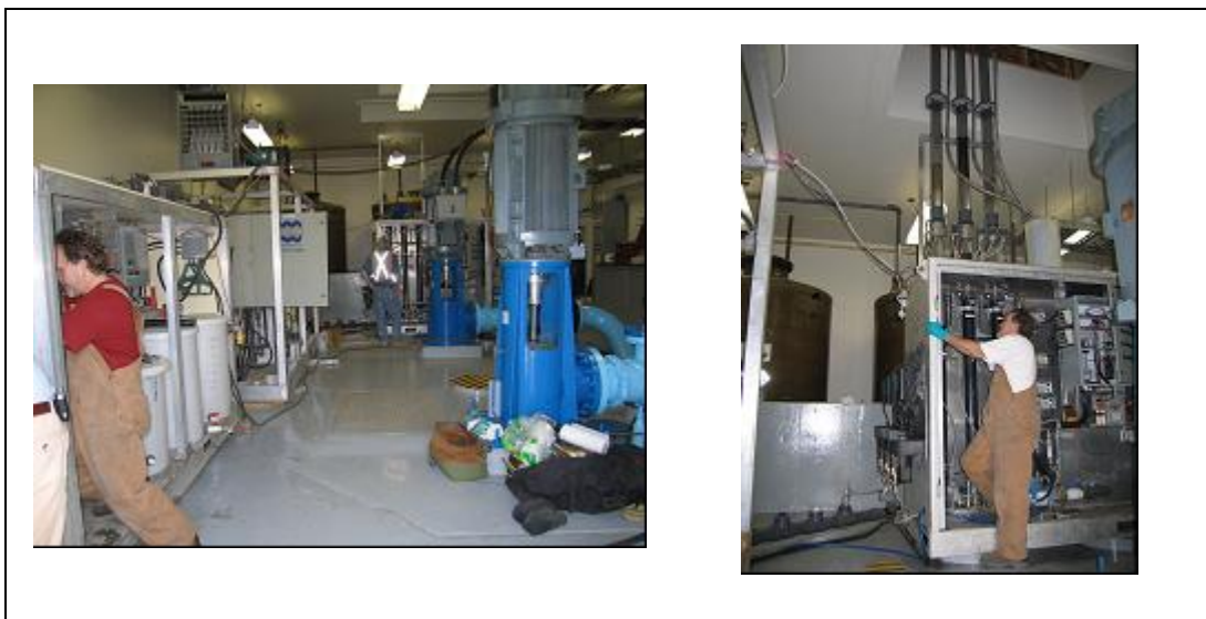
Figure A.1 Pilot-Scale Equipment at the Canoe Beach Pump Station
