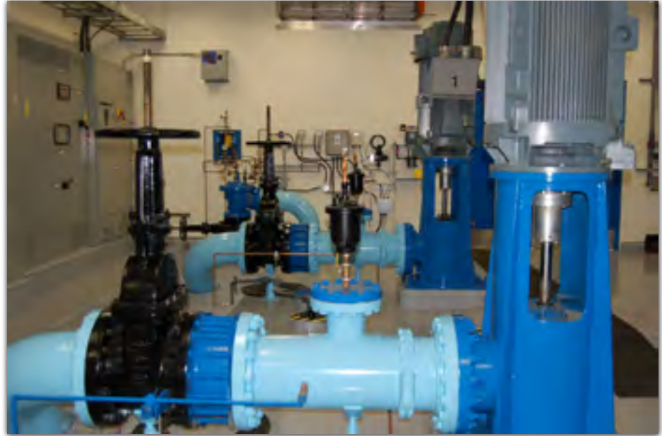
Figure 5 - Zone 1 Pumping Station at Canoe Beach
