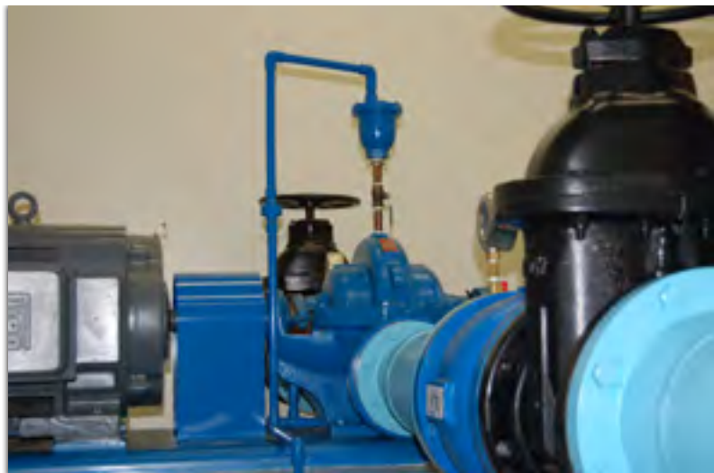
• Figure 6 – Zone 4 Pump/Pressure Reducing Station on 30th Street NE
