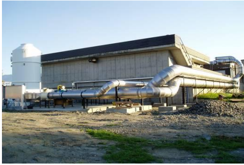
Single Stage Chemical Scrubber
