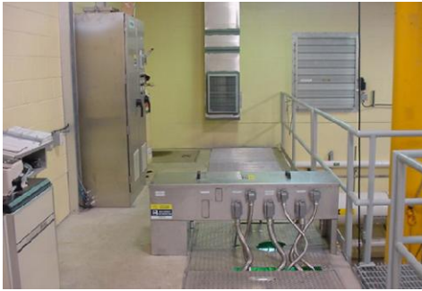
UV Treatment System
