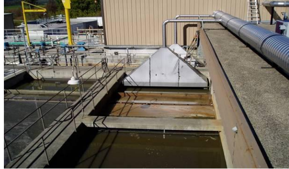
Primary Sedimentation Tanks
