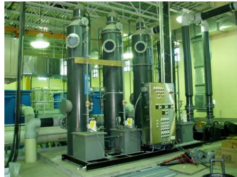
Train B Odour Scrubber
