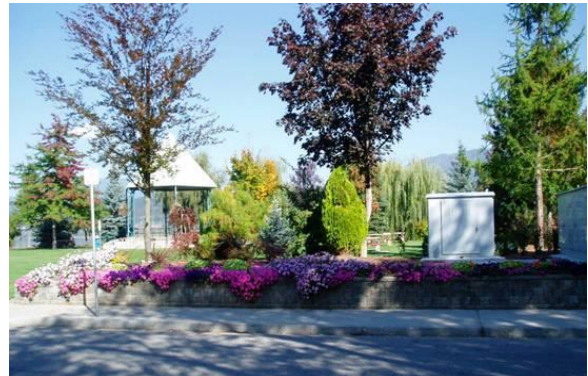
Wharf Street Lift Station
