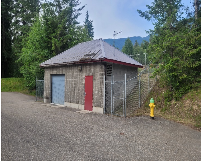
Zone 2B Booster Stn. 5160 40 th Ave. NW
