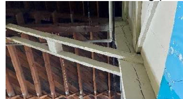
Photo 38.2 Typical knee brace.
