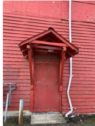
Photo 22: Hollow steel door
