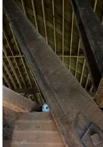
Photo 35: Web member with checking along entire length.
