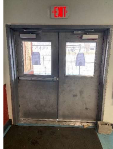
Photo 20: Insulated steel door
