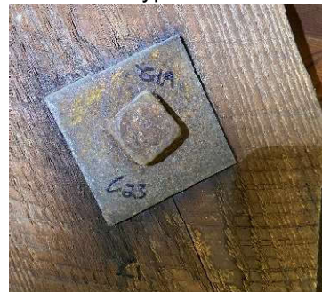
Photo 39: Typical surface corrosion on connection hardware.
