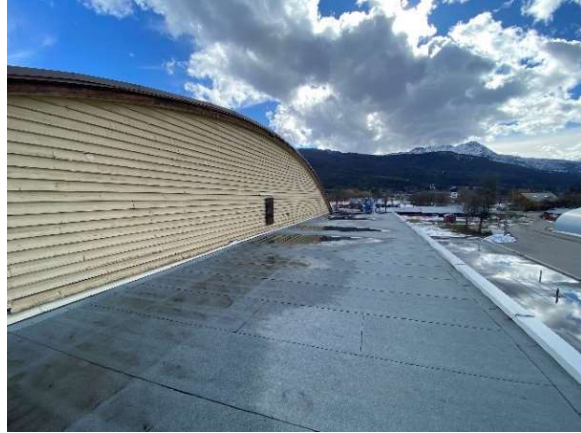
Photo 3: Flat roof at west end of arena. Ponding water observed.
