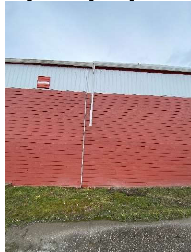
Photo 11: Typical condition of Hardi-plank lap siding.
