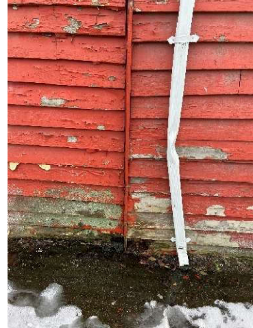
Photo 9: Cedar lap siding severely deteriorated within 48" of grade.
