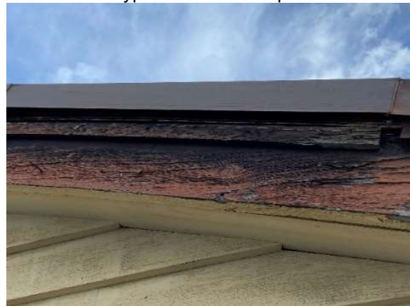
Photo 16: Deterioration present on painted facia board.
