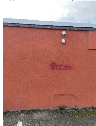
Photo 14: Typical condition of stucco siding.
