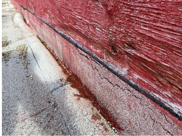
Photo 7: Microcracking, bond failure, and blistering observed.
