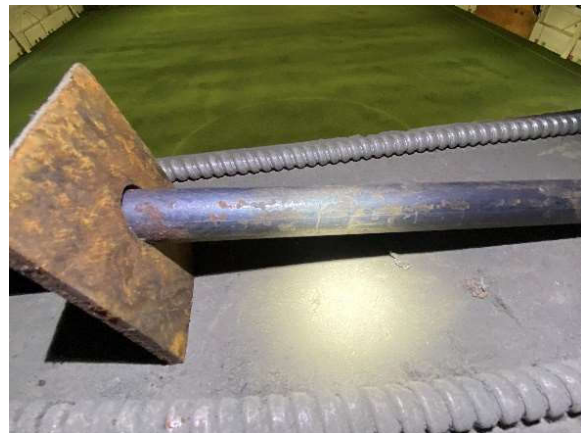
Photo 40: Typical bolt surface corrosion.
