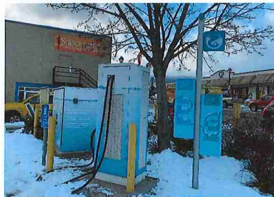
Electric Vehicle Charging Stations Ross Street Parking Lot
