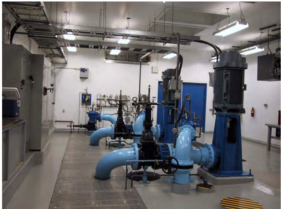
Figure 5 - Zone 1 Pumping Station at Canoe Beach
