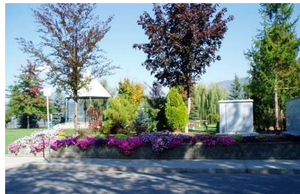
Wharf Street Lift Station
