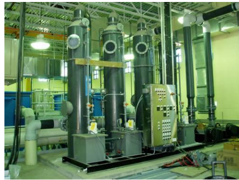
Train B Odour Scrubber
