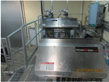
UV Treatment System
