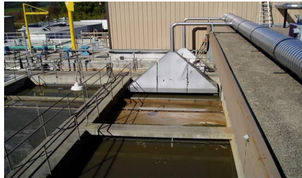
Primary Sedimentation Tanks
