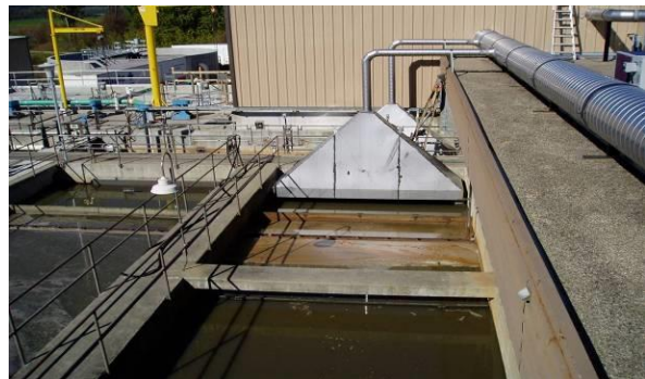
Primary Sedimentation Tanks
