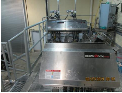
UV Treatment System
