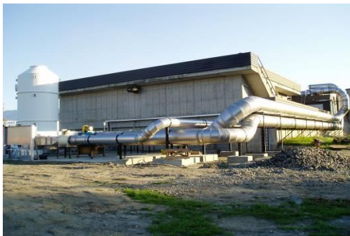
Single Stage Chemical Scrubber
