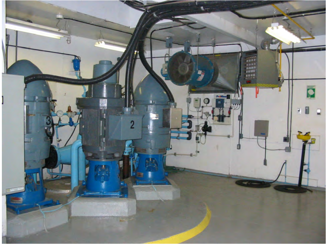
Figure 5 - Zone 2 Pumping Station at Canoe Beach
