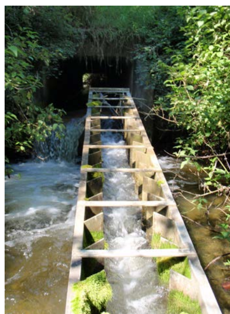
Figure. 2 Fish ladder for Trans-Canada Hwy crossing, stream segment # 10
