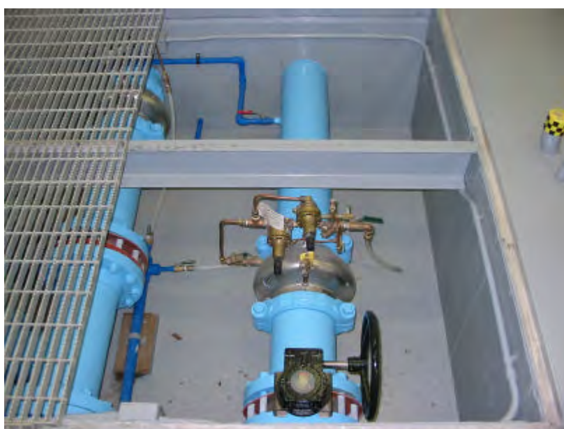
Figure 6- Pressure Reducing Station on 30 th Street NE.
