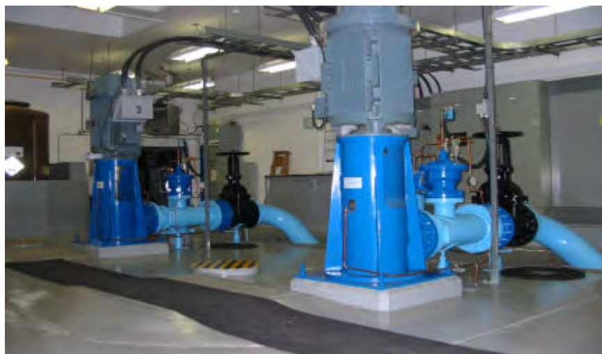
Figure 4 - Zone 4 Pumping Station at 30 th Street NE.
