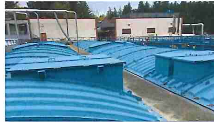
Covers on Primary Tanks help contain foul air
