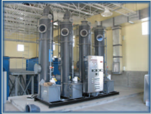
ATAD 4-stage Scrubber
