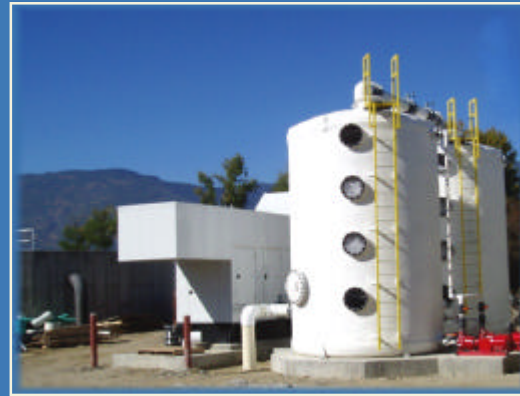
Bioscrubber and Ozone Contact Tanks
