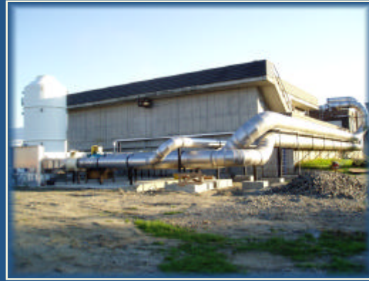
Main Plant Scrubber
