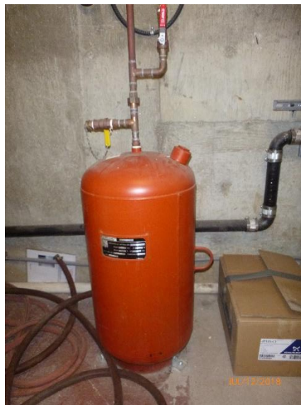
Figure 45 DHW expansion tank
