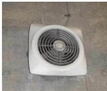
Figure 79 DE Filter Room Exhaust Fan
