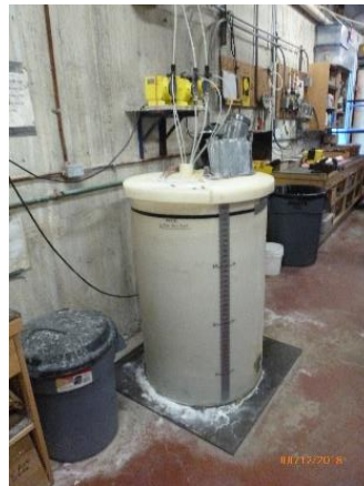
Figure 51 Soda Ash Container
