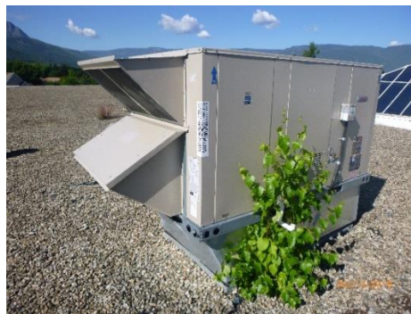
Figure 74 Pool Lobby RTU
