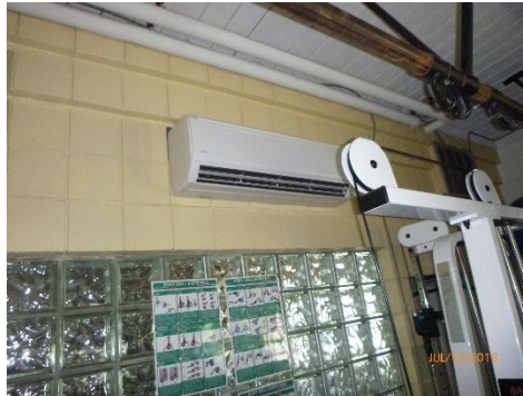
Figure 76 Gym's Split A/C unit
