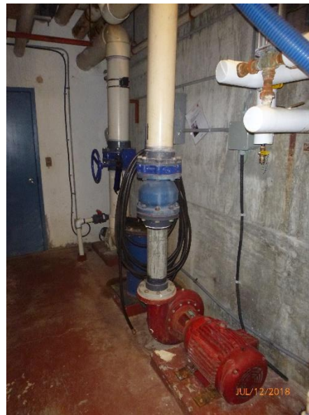
Figure 62 Hydro Air Pump
