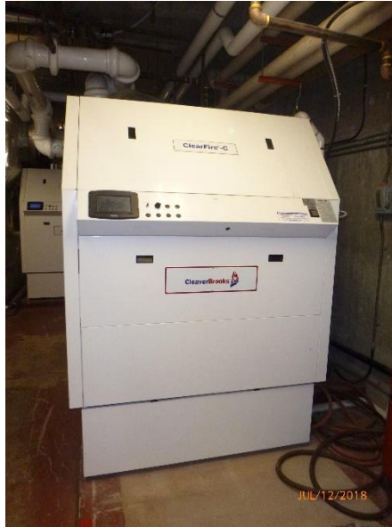
Figure 64 Existing Condensing Boilers
