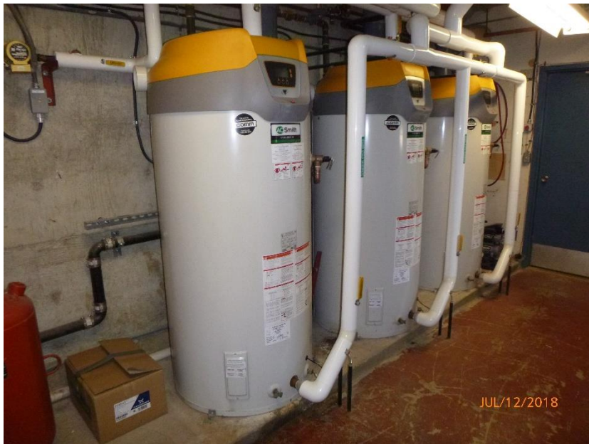
Figure 43 Domestic Hot Water Heaters
