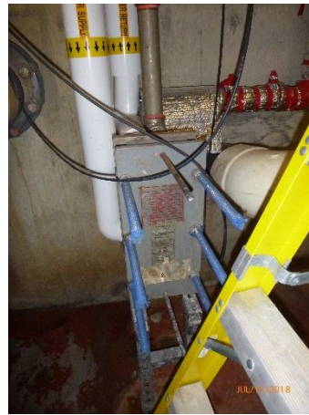
Figure 55 25m Pool Heat Exchanger
