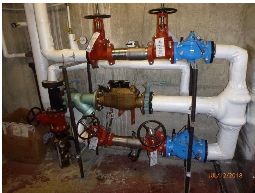
Figure 41 Water Entry Station
