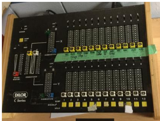
Figure 28: Defunct Stage Lighting Controls
