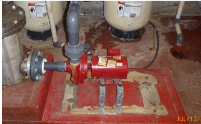
Figure 57 Main Circulator Pump
