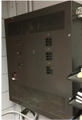
Figure 26: Existing Lighting control panel
