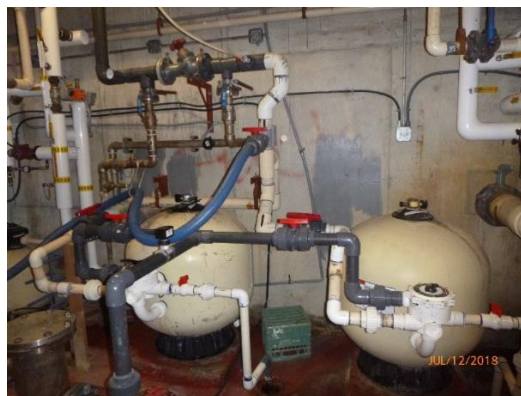
Figure 60 Wading Pool's Sand Filters
