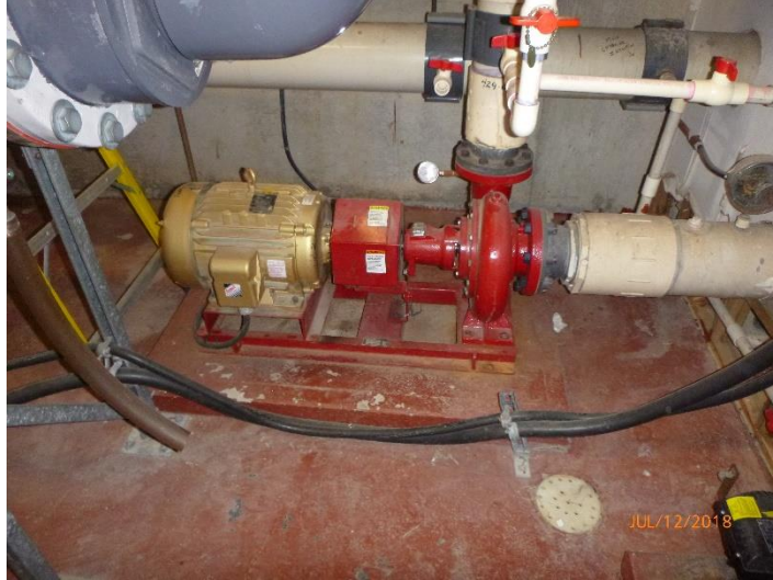
Figure 53 25m Pool's main Circulator Pump
