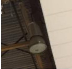
Figure 17 Gymnasium highbay light
