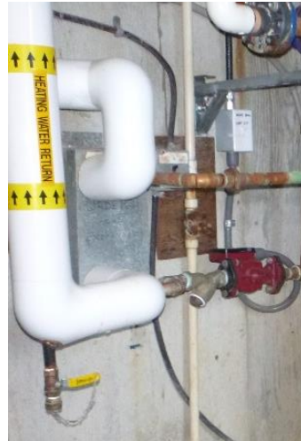
Figure 59 Wading Pool's Heat Exchanger
