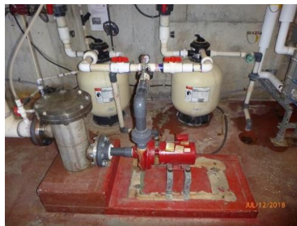
Figure 56 Wading Pool's Sand Filters
