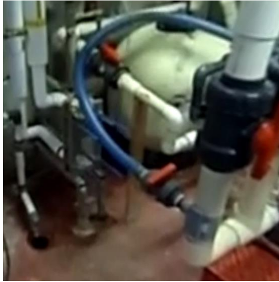
Figure 63 Wading Pool's Heat Exchanger
