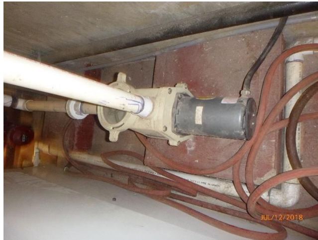
Figure 58 Fountain Re-circulation Pump
