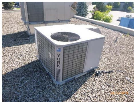
Figure 75 Lv.2 Office A/C
