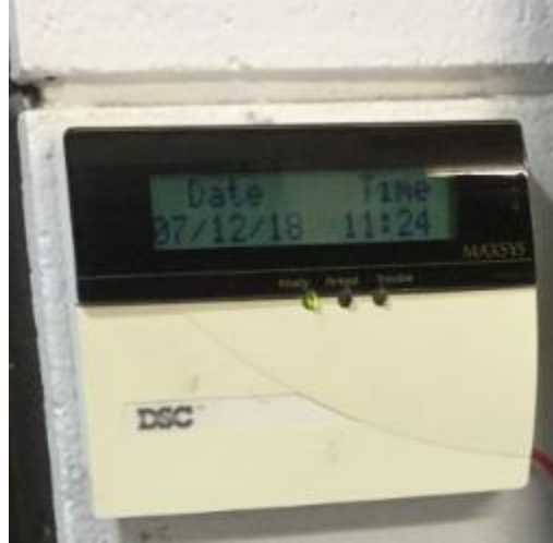
Figure 34: Existing security control panel
