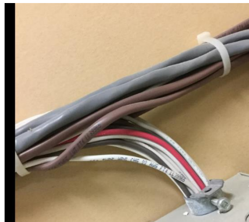
Figure 40: Sample Existing FT4 cable
