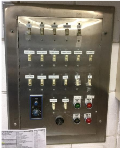
Figure 29: Manual control switch bank
