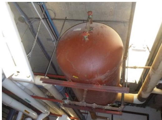
Figure 67 Ex. Expansion Tank
