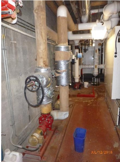
Figure 66 Main Circulator Pumps
