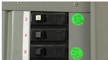
Figure 2: Sample pool lights, not GFCI
