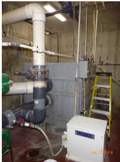
Figure 50 DE Tank and DE Feeder
