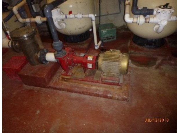
Figure 61 Main Circulator Pump
