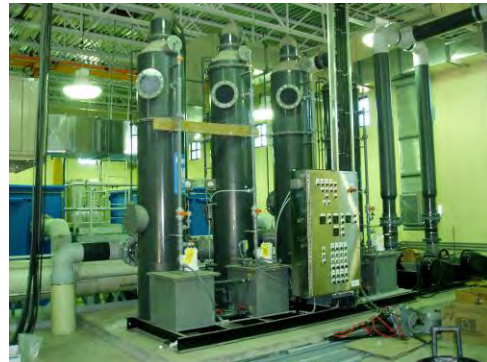
Train B Odour Scrubber
