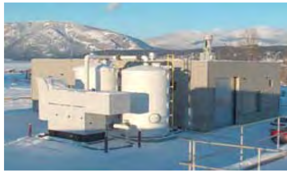
Generator Set, Train B - Odour Control and Filtration Building
