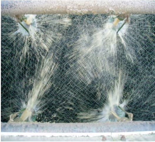
Old Splash Plate Nozzles with unequal distribution
