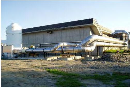
Single Stage Chemical Scrubber
