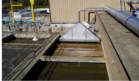
Primary Sedimentation Tanks
