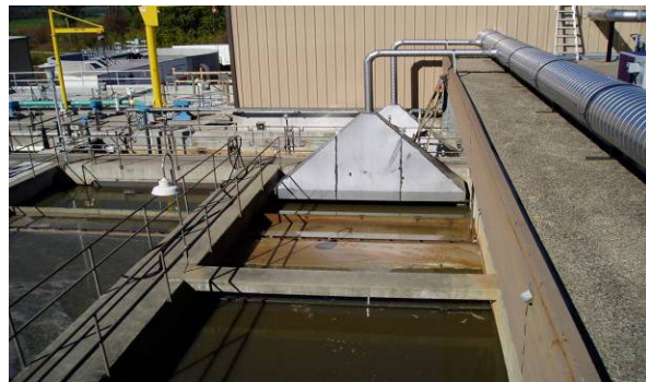
Primary Sedimentation Tanks
