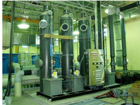
Train B Odour Scrubber
