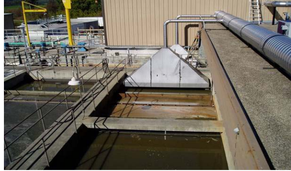
Primary Sedimentation Tanks
