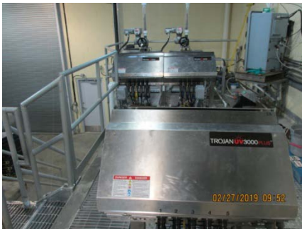
UV Treatment System
