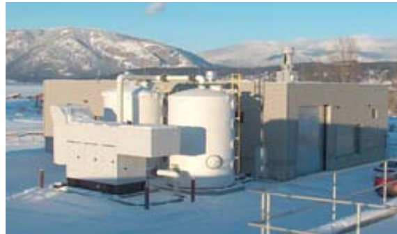
Generator Set, Train B - Odour Control and Filtration Building
