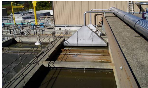
Primary Sedimentation Tanks
