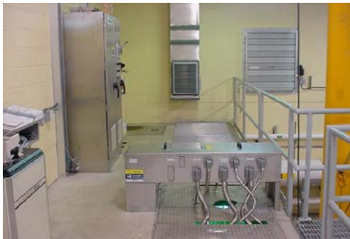
UV Treatment System
