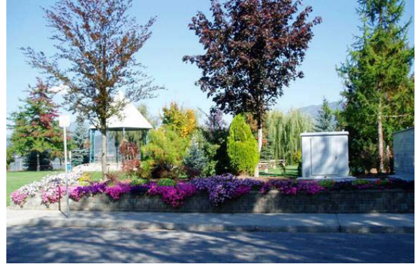
Wharf Street Lift Station
