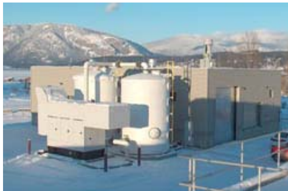
Generator Set, Train B Odour Control and Filtration Building
