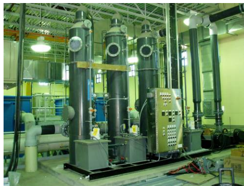
Train B Odour Scrubber
