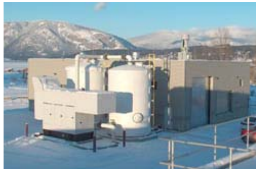
Generator Set, Train B – Odor Control and Filtration Building
