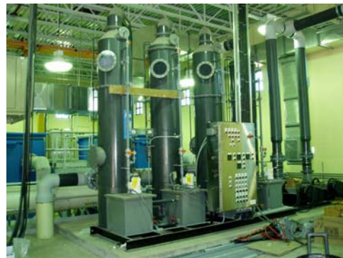
Train B Odour Scrubber
