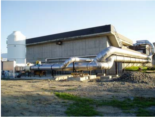
Single Stage Chemical Scrubber
