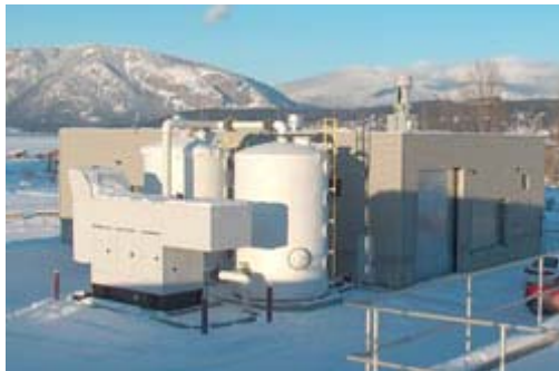
Acoustic Housing, Generator Set, Train B – Odor Control and Filtration Building
