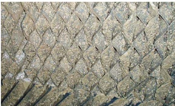
Cross flow Media prior to sloughing
