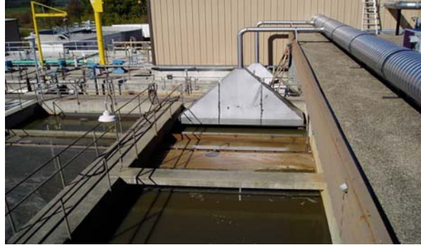
Primary Sedimentation Tanks
