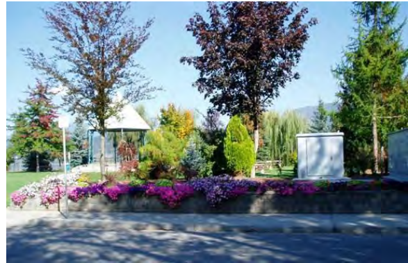
Wharf Street Lift Station
