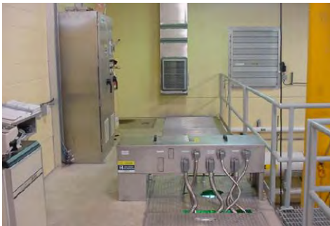
UV Treatment System
