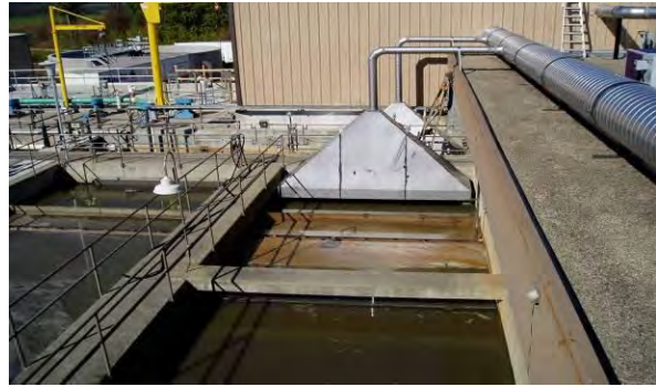
Primary Sedimentation Tanks
