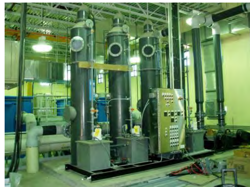
Train B Odour Scrubber
