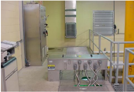
UV Treatment System
