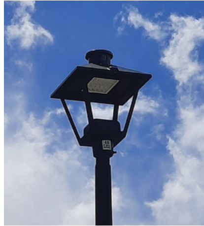
New residential LED lighting
