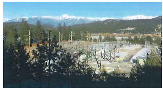
Located in Cranbrook's industrial area, Joseph Creek Substation is undergoing a $17 million upgrade. Photo courtesy of Sally Masters
