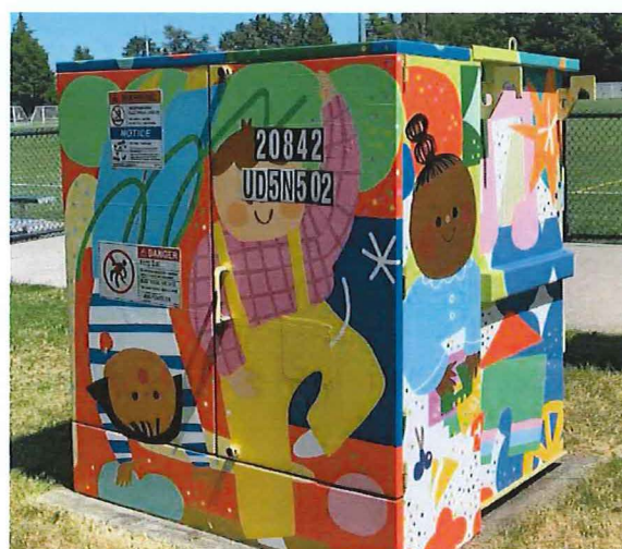
Example of a decorative wrap added to BC Hydro equipment. Photo courtesy of the City of Richmond.
