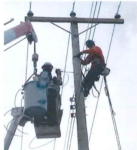
BC Hydro crews restoring electrical infrastructure in the Village of Lytton in January 2023. Photo courtesy of Clay Rhodenizer
