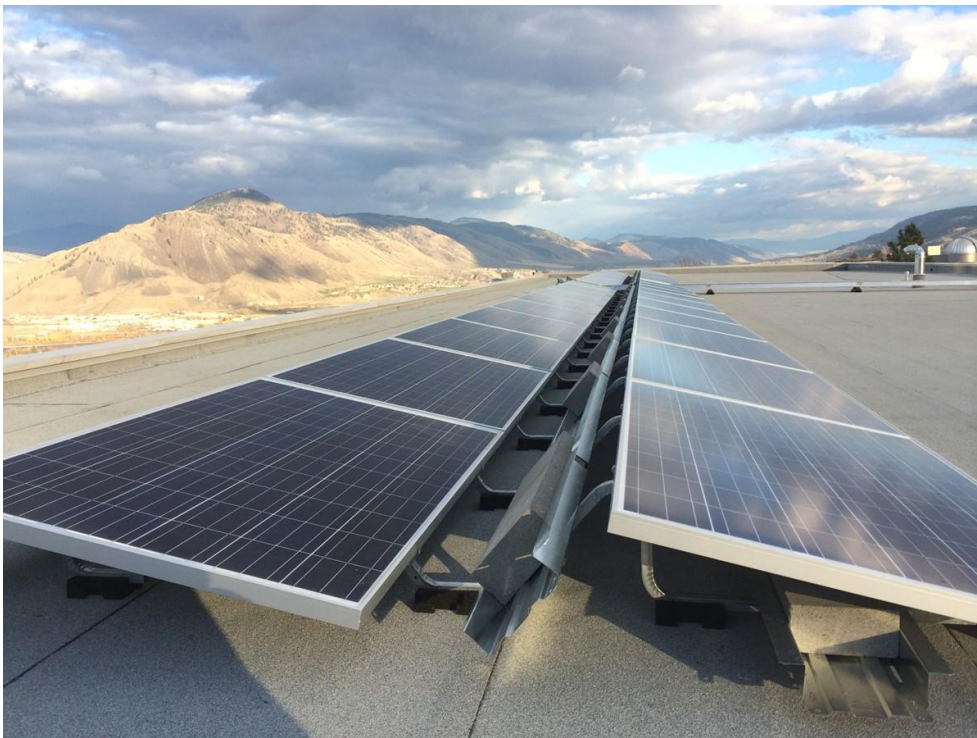
10.2 kWp Array using Ballasted Racking – Thompson Rivers University, Kamloops BC
