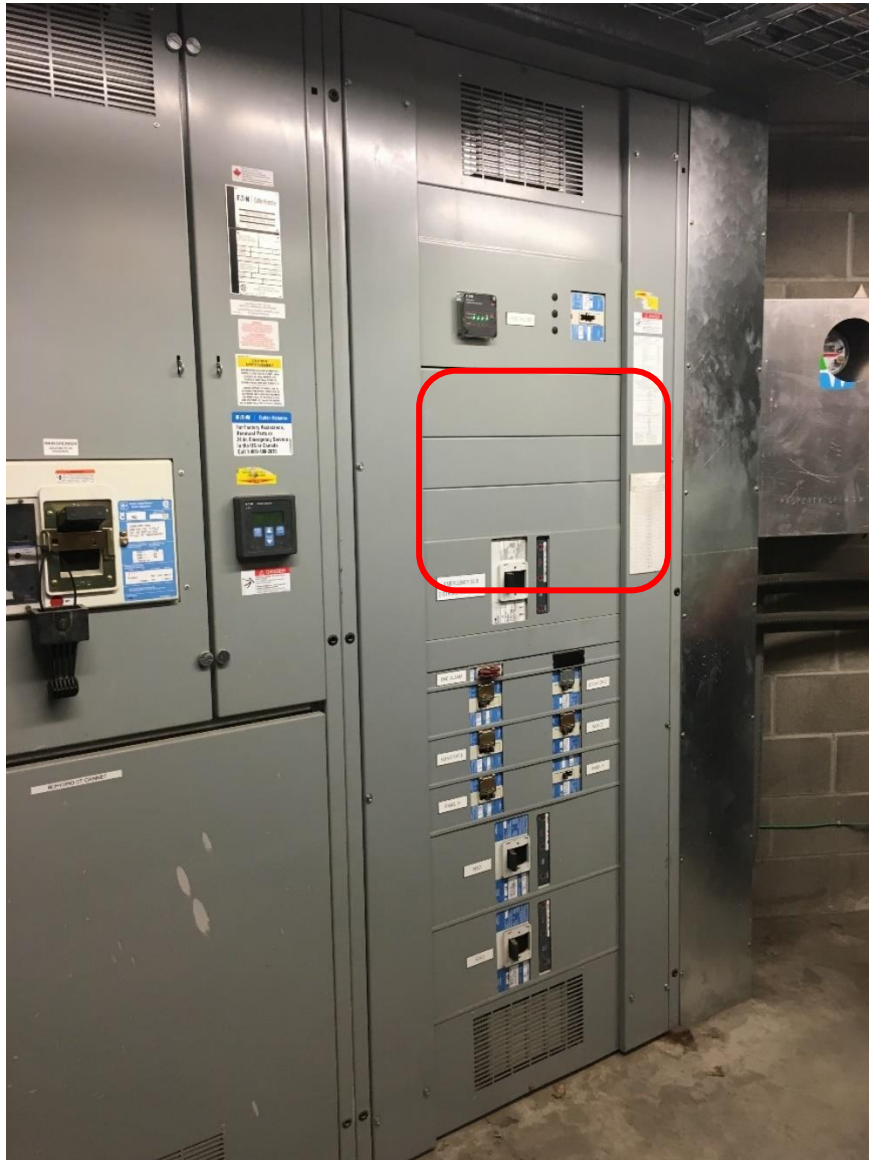
Figure 21: MDC - Room 004 – Spare Breaker Positions
