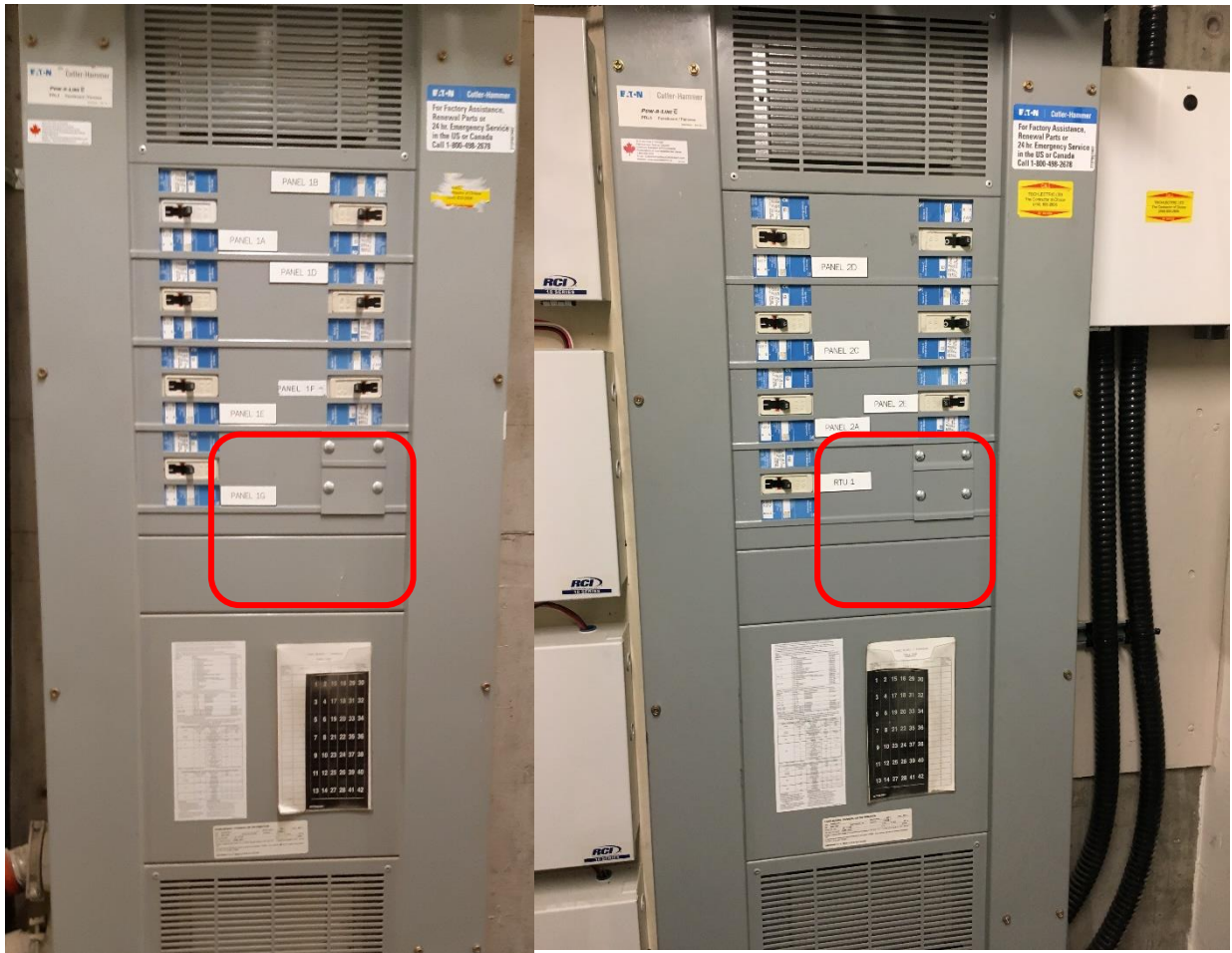
Figure 22: SDC1 (Room 138) and SDC2 (Room 226) Spare Breaker Positions
