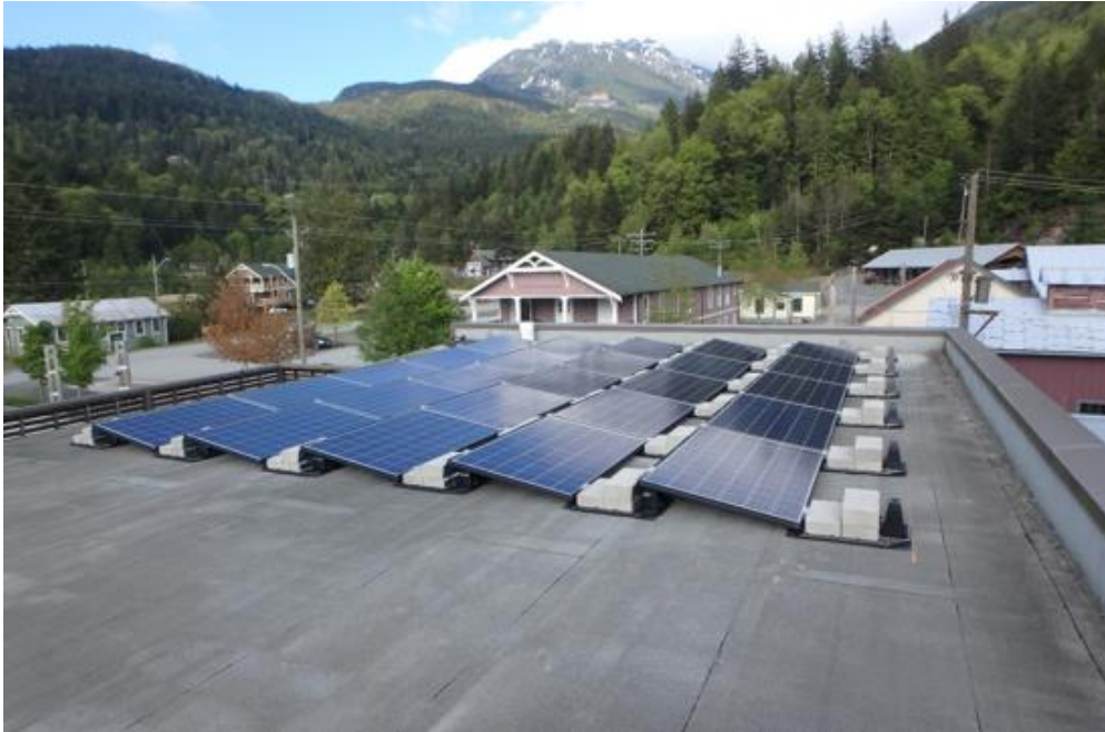
6.4 kWp Array using Ballasted Racking – Britannia Mine Museum, Britannia BC
