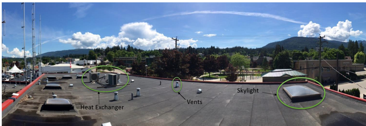
Figure 32: Fire Hall No.3 South Roof Obstructions
