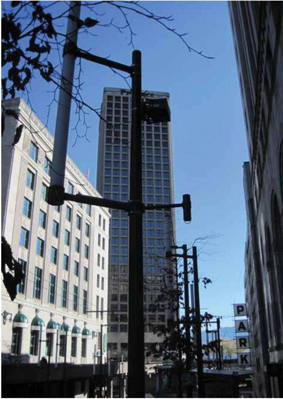
Small cell attachments to decorative street lights (the white vertical element is the light)
