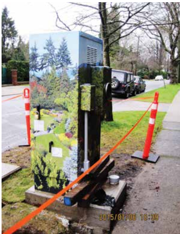
Close-up of connection cabinet
